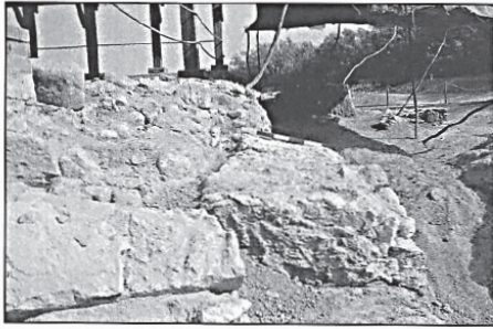
4. The bedding of the central aisle settled about 30 centimeters (from the south).
